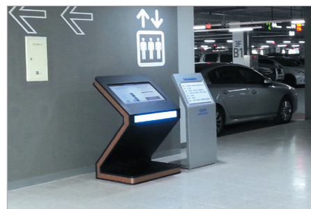
Parking Guidance System
